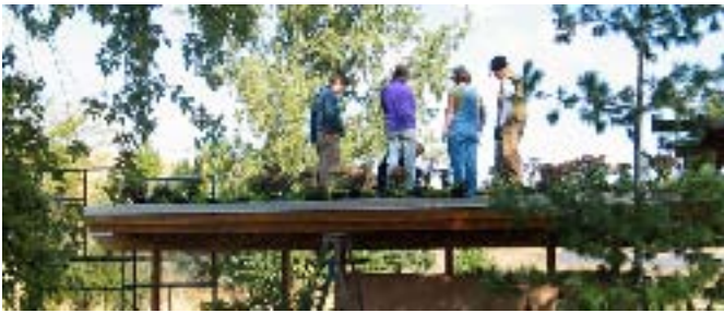
Volunteers watch as the correct planting technique for living roofs is demonstrated. Photo: Aly Bean
