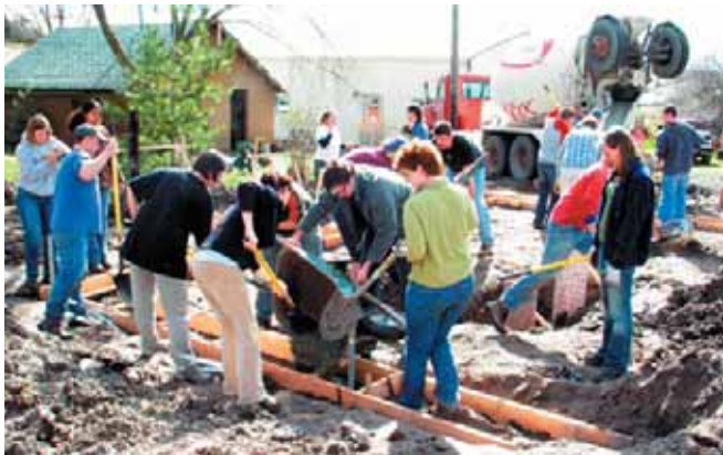
Many hands make light work of all that concrete. Photo: Kelly Riley
