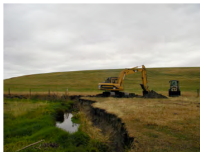
October 2006: Newly constructed point bar. The restoration plan was designed to mimic the natural meanders of the creek. Stream bank slopes were resloped to a minimum 3:1 in most places.
