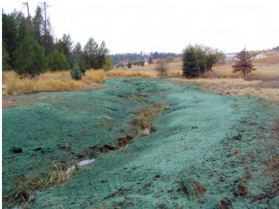
October 2007: Hydro-mulching was used on site to help increase seed germination rate and to help stabilize banks following excavation activities.
