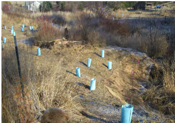
October 2007: Steep banks throughout the project extent were resloped and stabilized with hydro-mulch and erosion control fabric. Following stabilization activities the site was planted with native trees and shrubs.
