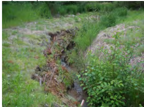
August 2010: Brush revetment installed to reduce active in-stream erosion in areas on the bank that were difficult to access with excavating equipment.
