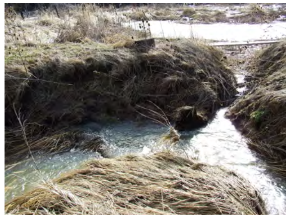
February 2006: Lack of riparian vegetation has lead to the sloughing of the bank in many areas along the project reach.
