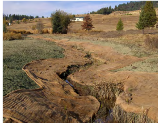
October 2007: Photo point 3 upstream. Pos-construction banks were hydro-seeded with native grasses. Erosion control fabric helps stabilize banks.
